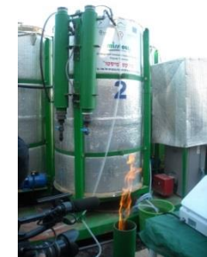
Digesters on a platform, and next to them the heating system, and in front the Methane burning
